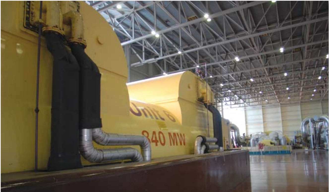
The turbine hall in the Bruce B generating station.
