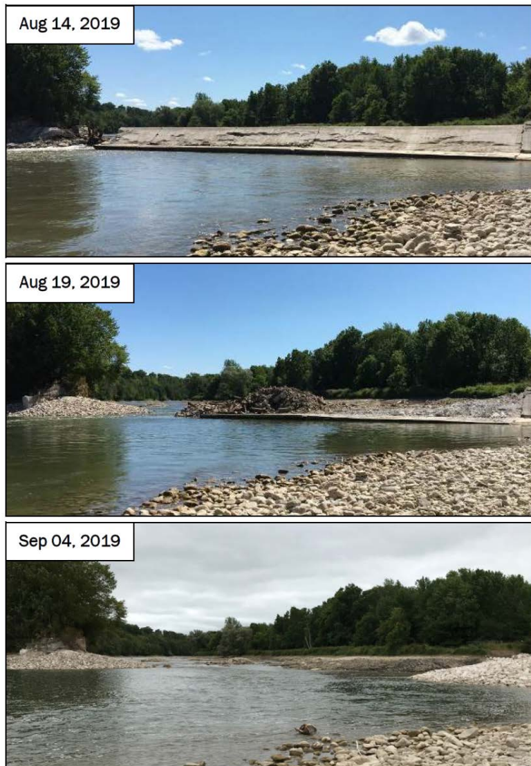
Figure 60 - Truax Dam, Walkerton, ON. The original wooden dam was built in 1852 and later replaced by the concrete structure shown above in 1919. The dam posed a significant barrier to fish passage for more than a century before it was removed in the summer of 2019 over the course of 3 weeks
