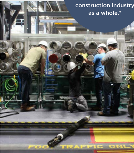
Millwrights and Boilermakers in a replica of the vault. For three weeks, they trained on the specialized tooling before moving to site for the first Major Component Replacement project of Unit 6 (MCR6).
